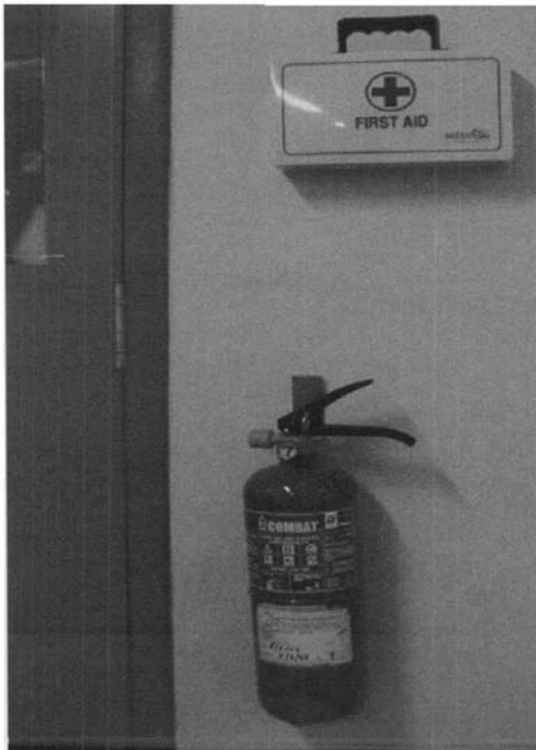
Fig. A.6 Safety kit and fire extinguisher.
