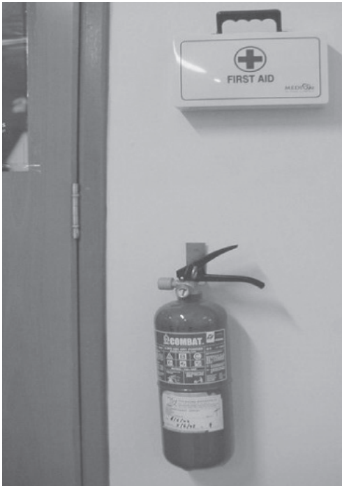
Fig. A.6 Safety kit and fire extinguisher.
