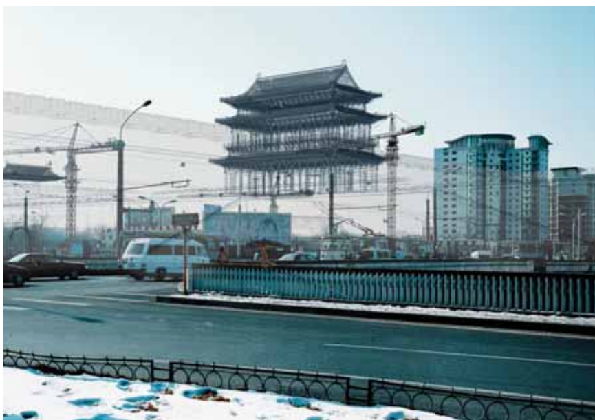
An artist's rendition of Beijing's Chaoyangmen area and the demolished Chaoyangmen Gate (by courtesy of Beijing Crystal Digital Technology Co. Ltd.)
